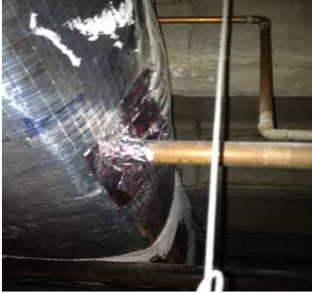
Pipe penetrating supply air duct in return fur down above first floor tenant ceiling.
